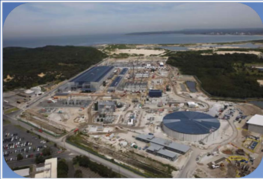
Aerial view of the $2bn Kurnell Desalination Plant under construction while Sydney's dams fill up
